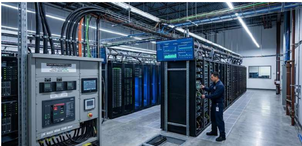
Fig 5.1: Data center operations and power management
